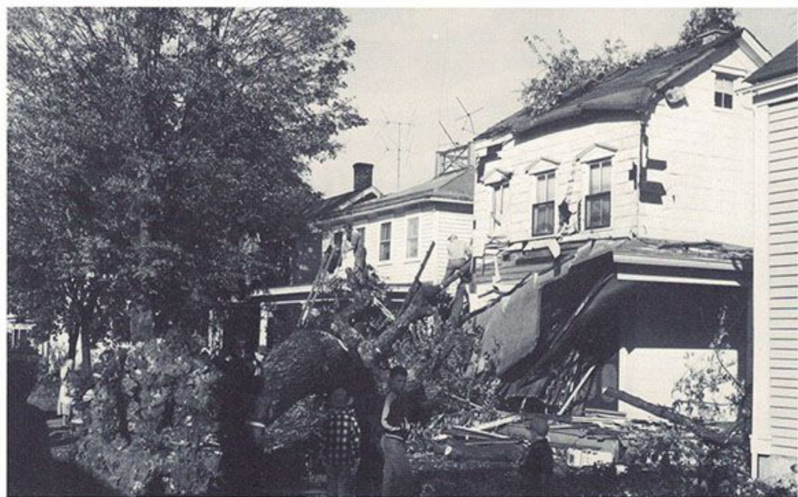
Oct. 1954, Hurricane damage to a dwelling on upper Third Street.
